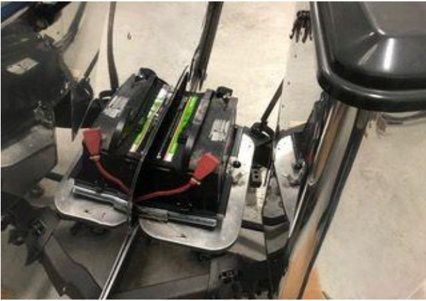
This is how far the battery slides out of the trailer for servicing.
